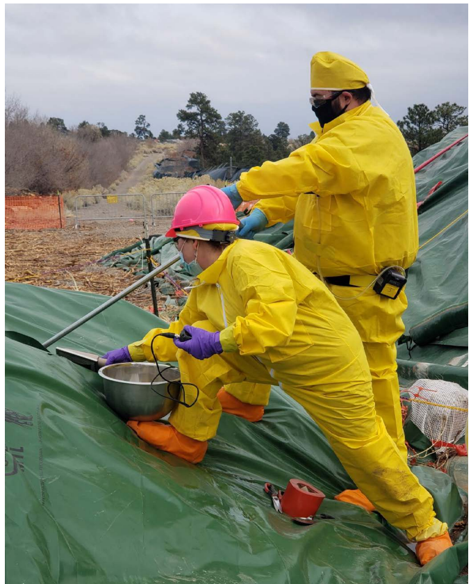
Middle Delta Prime Road Project, Los Alamos National Laboratory Soil sample collection activities on pile.
